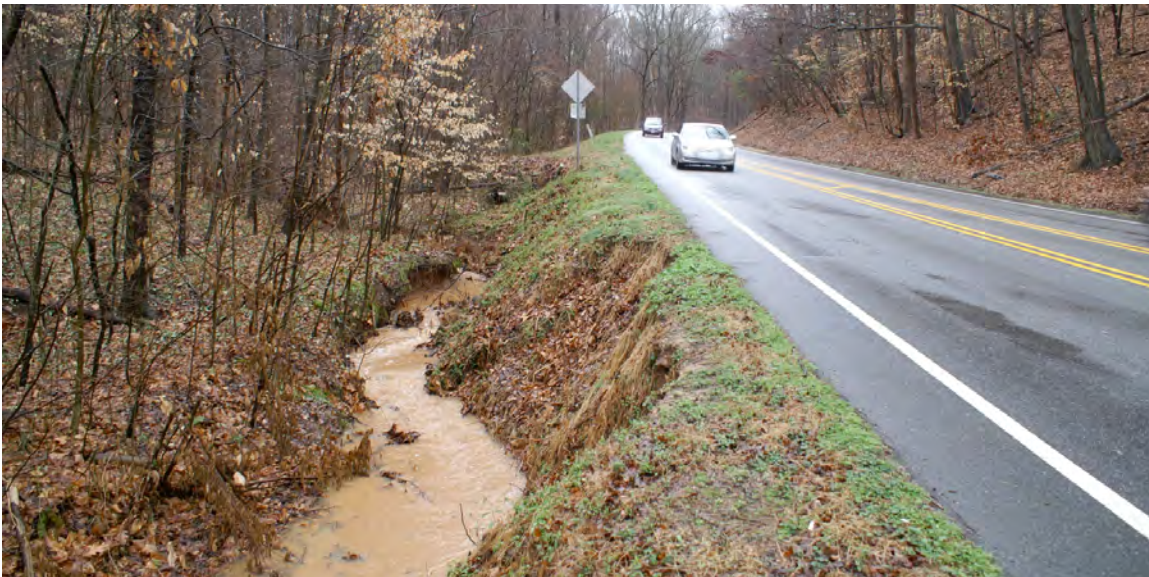
FIGURE 5: LATERAL INSTABILITY/STREAMBANK EROSION THAT IS THREATENING A ROAD.
