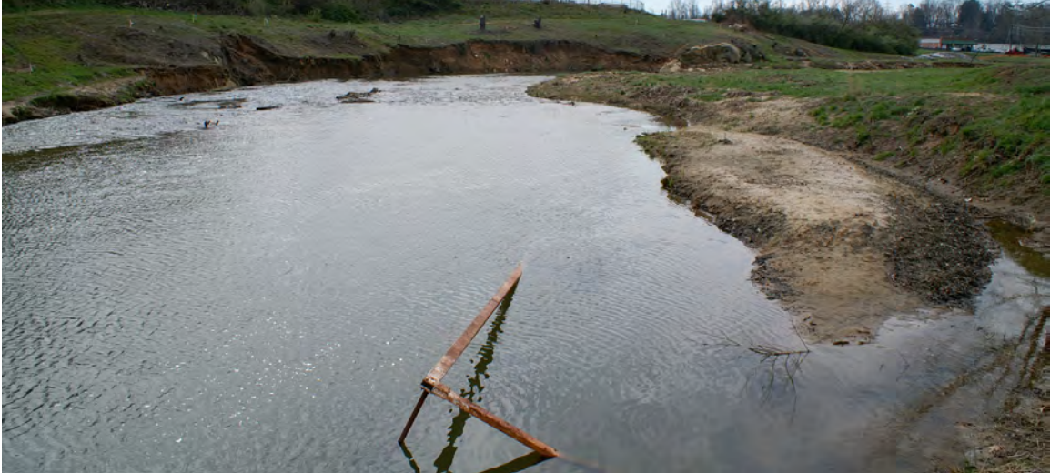
FIGURE 7: AN ERODING STREAMBANK ALONG A PREVIOUSLY DESIGNED FLOOD CONTROL CHANNEL
