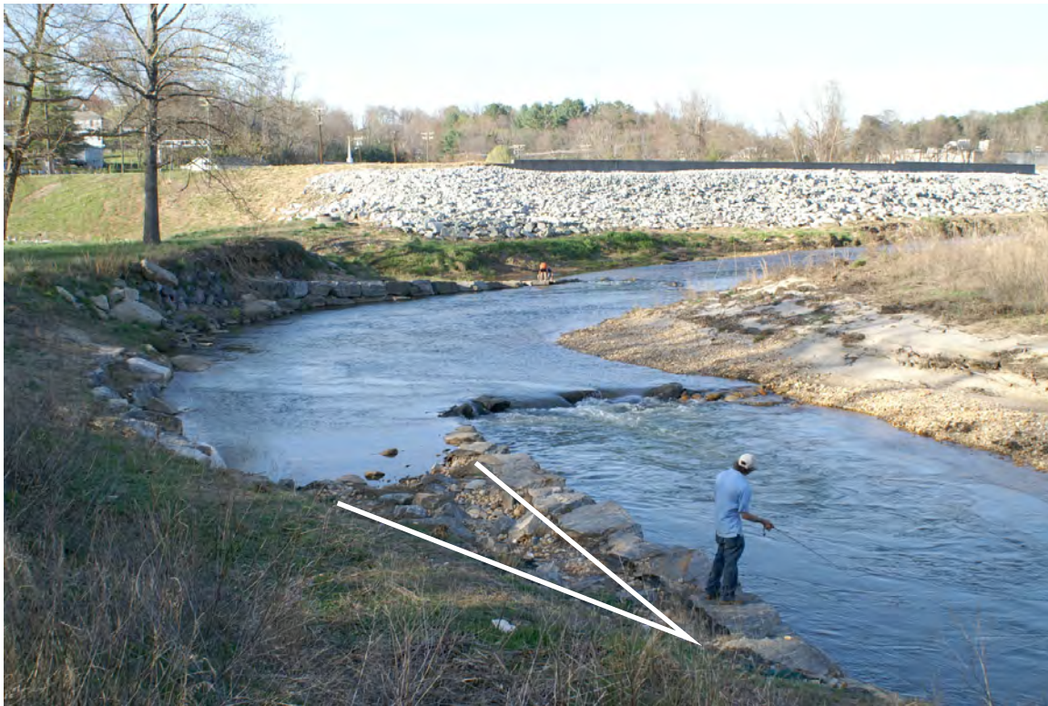
FIGURE 11: J-HOOK VANE AT BASE FLOW. The triangle is formed from the vane arm where the fisherman is standing and the streambank. The structure is placed downstream of where the velocity vector intercepts the bank.
