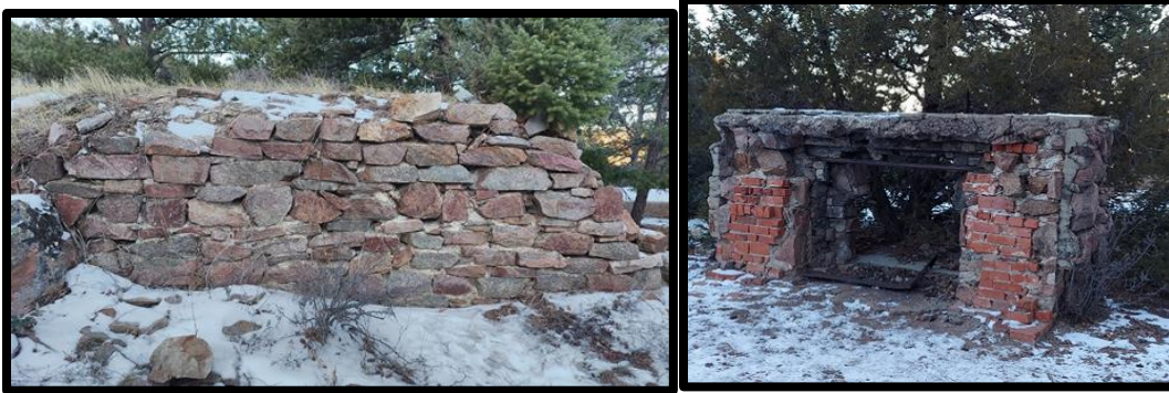
Figure 10. Crags Hotel ruins on Rattlesnake Trail December 2020. Visitors enjoy the view and exploring this area. Updated signs and possibly a “virtual tour” (this is one of the few spots in the Park with strong cell signal) would help promote the uniqueness of this site and encourage protection of structures that have been standing for over a century.
