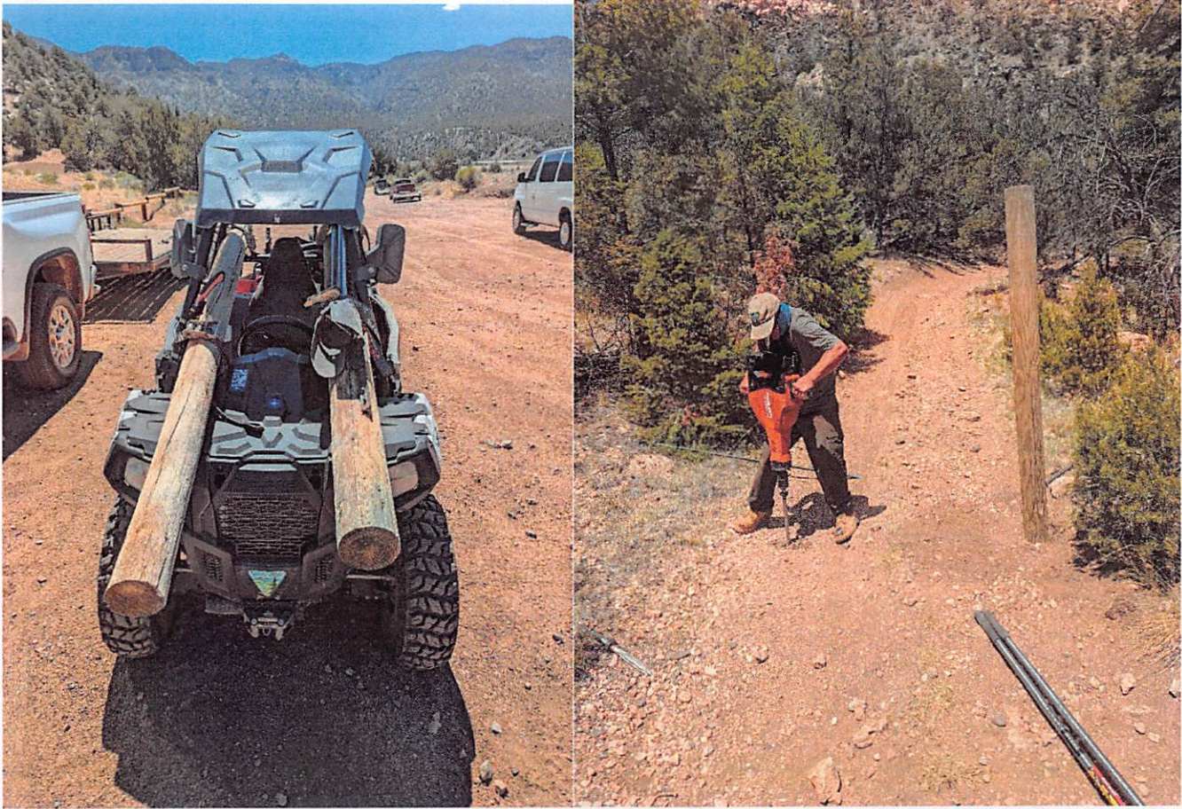
Image 1: Installation of 50" limiter at entrance to T6027A, per expectation of FY23 crew duties.
