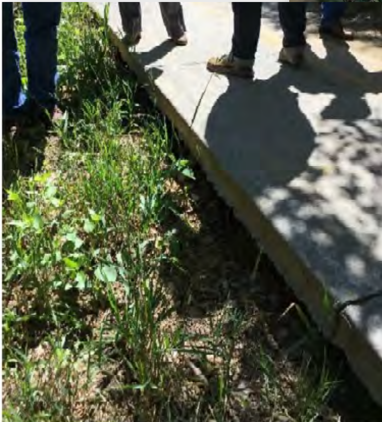
RIGHT: Erosion under trail. (2019 image)
