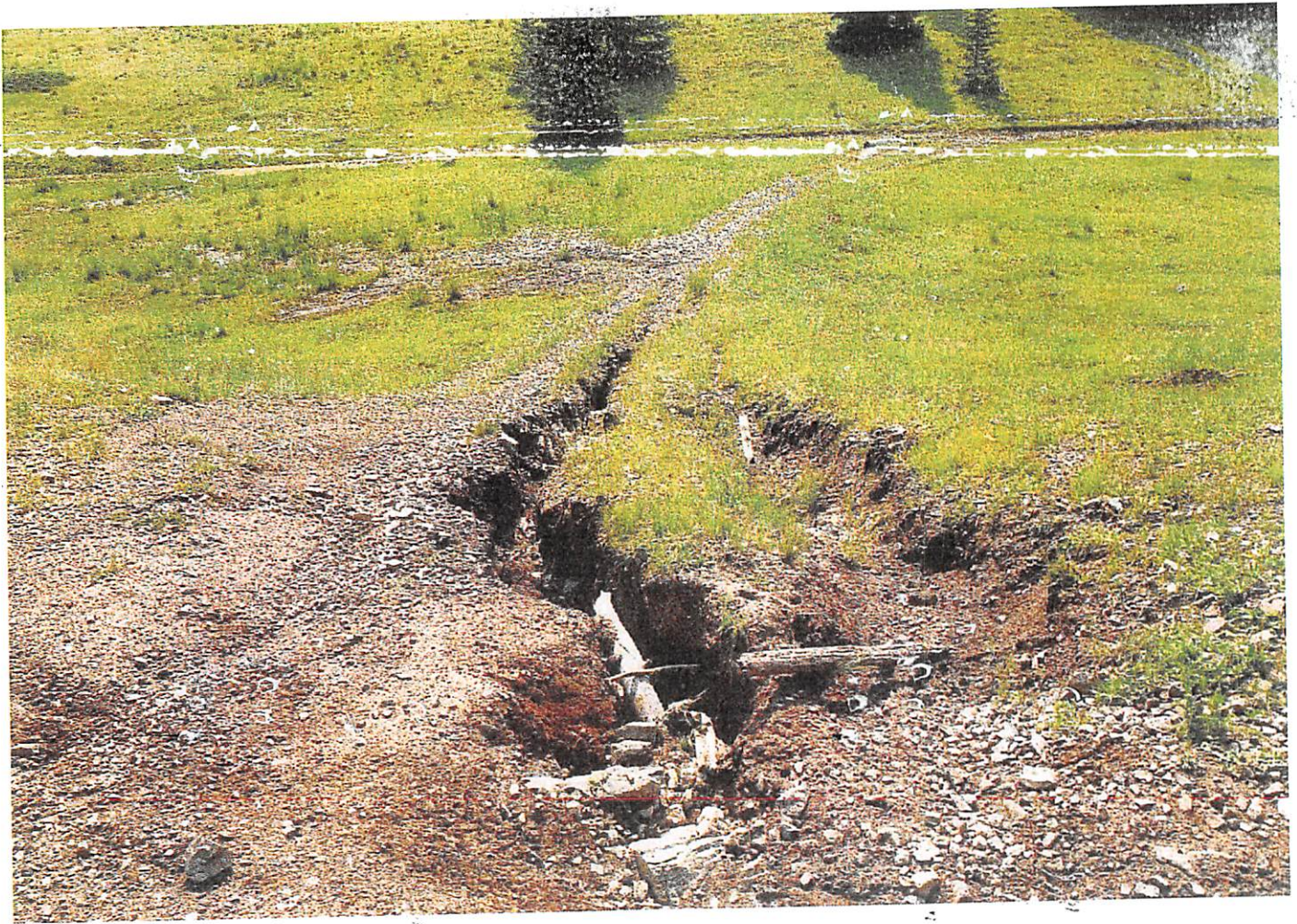
Rutted road due to drainage issues.
