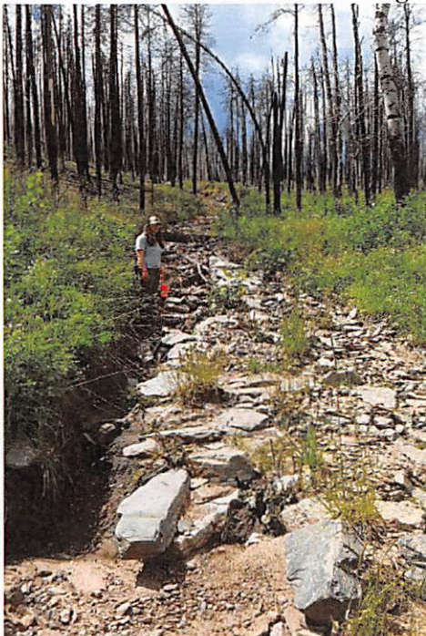
Photo 3: Storm Mountain drainage ditch repair needed (extensive quick capture date available)
