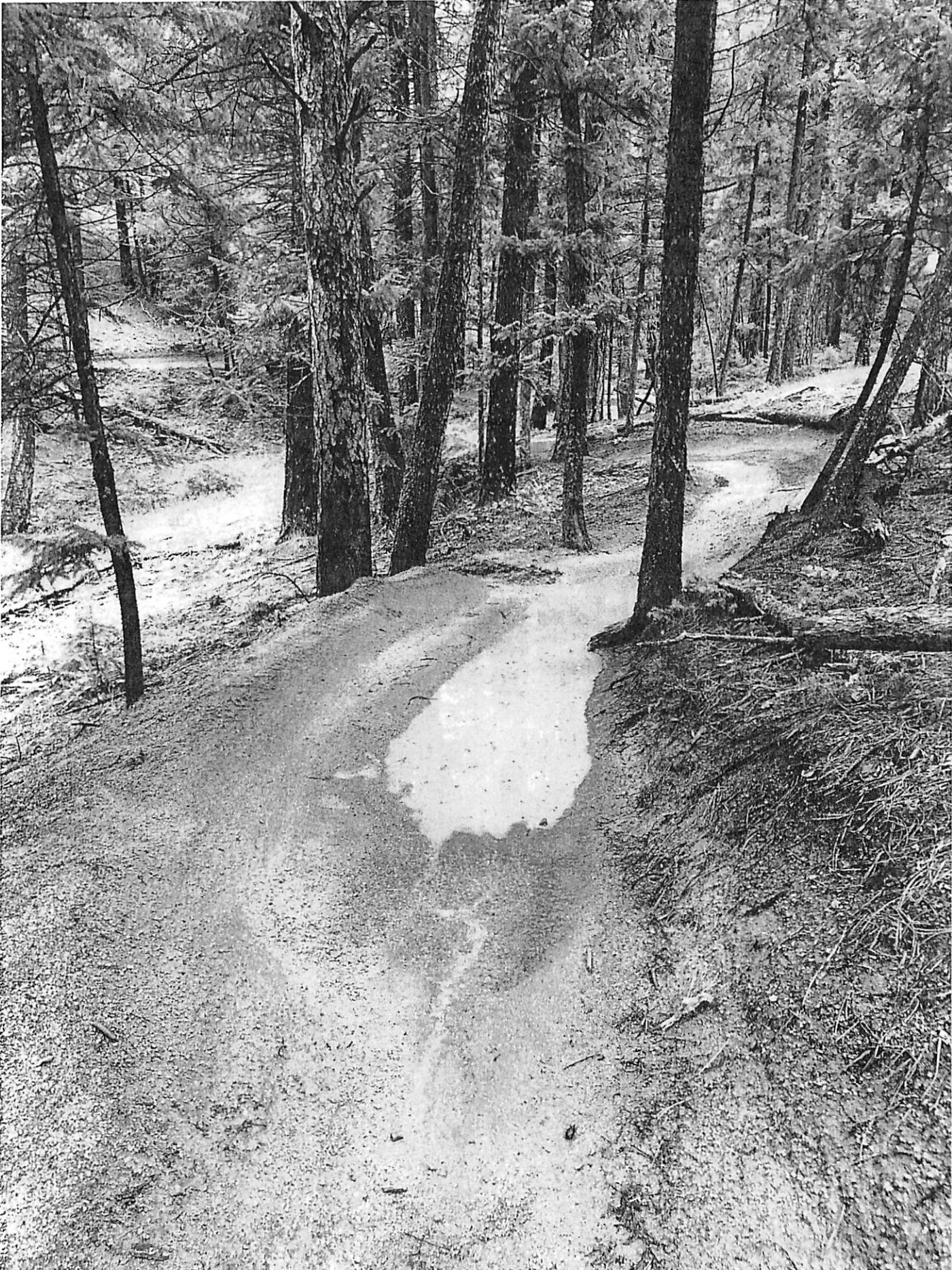
Typical drainage work needed
