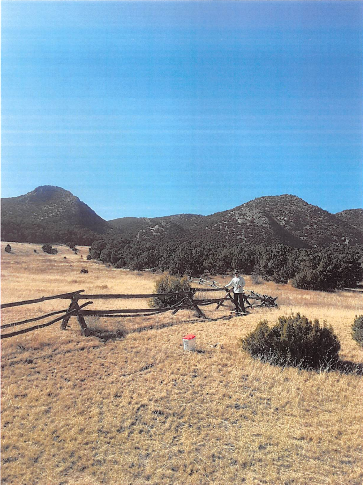
Image 2: Repairing buck and rail fence at Seep Springs to prevent off-route travel through vegetation.
