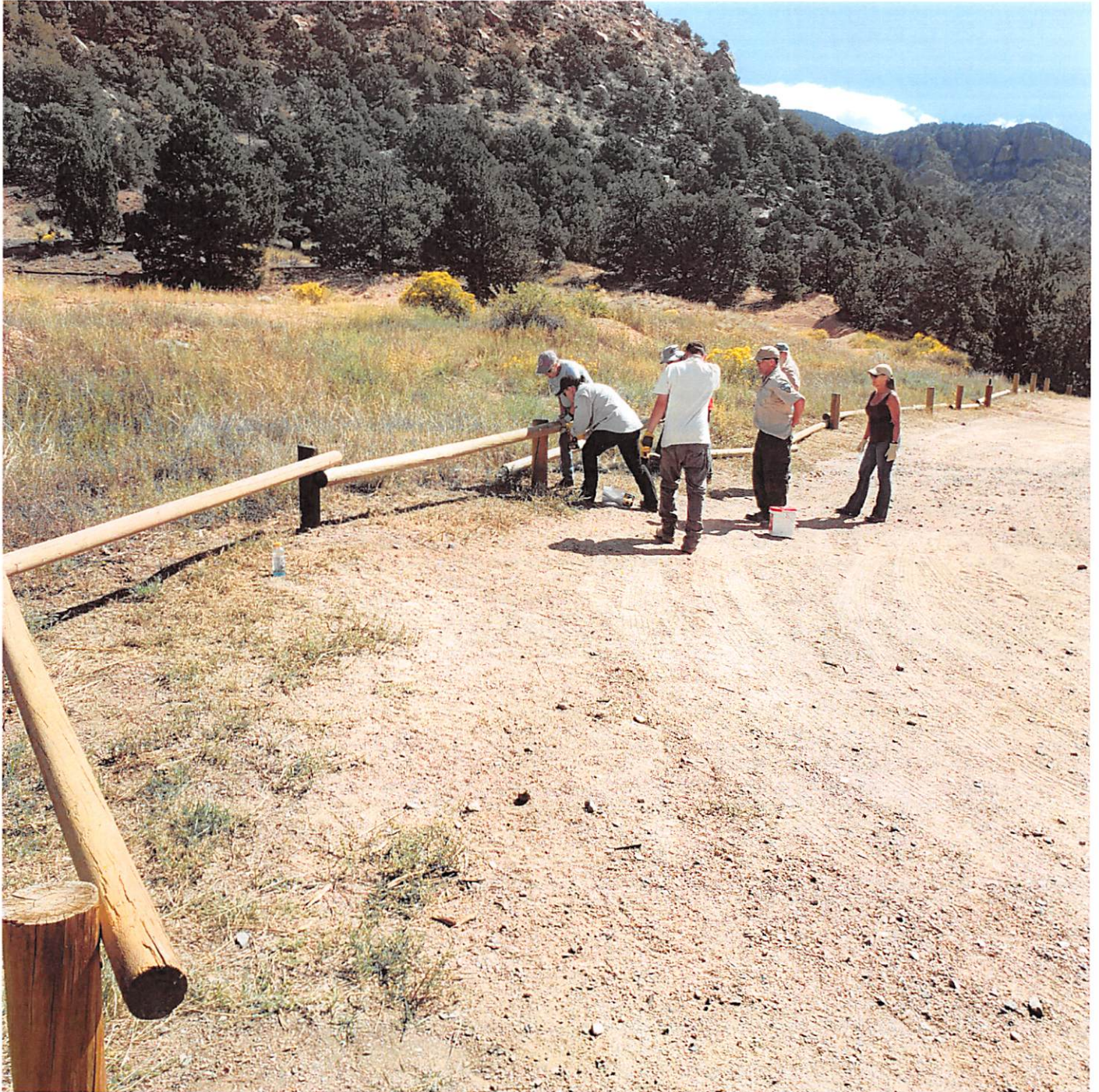
Image 3: Replacement of dilapidated fencing with new post and rail at Texas Creek. Volunteer support provided by Royal Gorge ATV Club.
