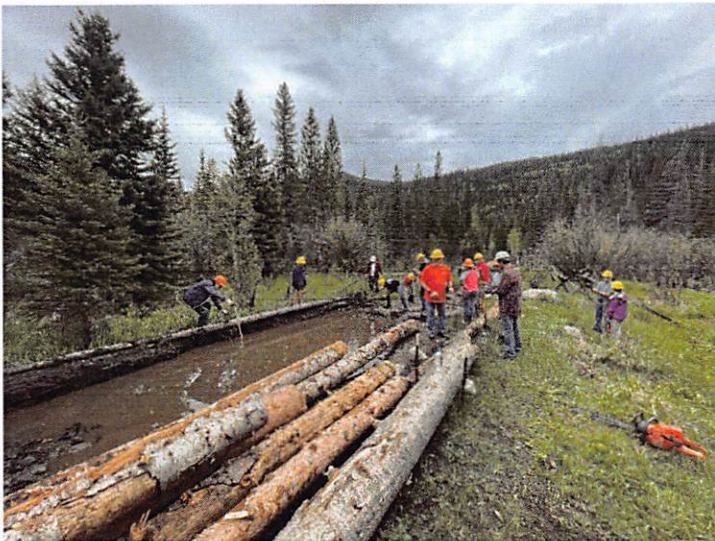
Left: Finished surface on Middle St. Vrain with volunteers adding final gravel fill to road tread. This vital work needs regular maintenance to protect the adjacent riparian area and nearby waterway.
