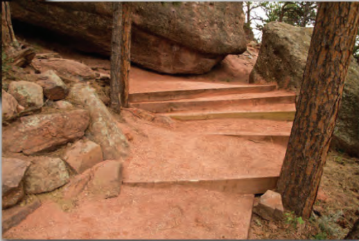
Below: 5 treated timber steps and 15 square feet of wall (up to 3 tiers) was installed to level the landing pad, slow down water and create a safer landing for the bouldering community.
