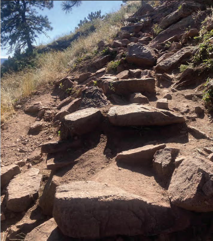
The East Ridge summit approach. Inadequate infrastructure for the grade and visitation.
