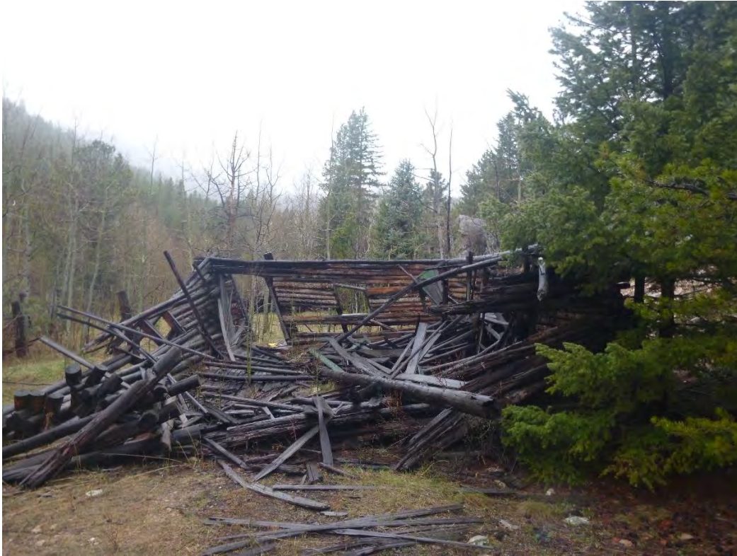
Photo 34. Phillips Ranch in May 2015: an example of structural collapse likely due to heavy snow and decay.
