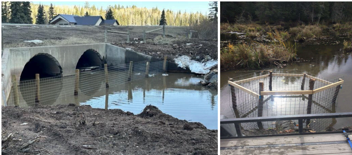
Left: Photo by Rory Cowie, Alpine Water Resources, LLC, Silverton, CO, showing two large concrete culverts protected from beaver damming by an exclusion fence. Right: Photo Best Management Practices for Resolving Human-Beaver Conflicts in Vermont (2017) showing a hexagon shape that has good success deterring beaver.
