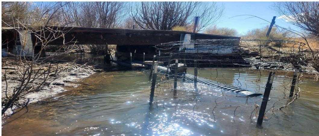
Photo provided by the RGNF of the pipe flow device that has been successful in keeping the water level below the bridge and road.
