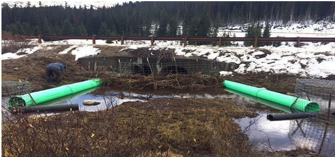
Photo of a double flow pipe and culvert exclusion fencing installed in 2018 by Summit County located adjacent to Highway 9 at Summit County's Monte Cristo Open Space near Quandary Peak. Photo by Summit County Open Space and Trails staff.
