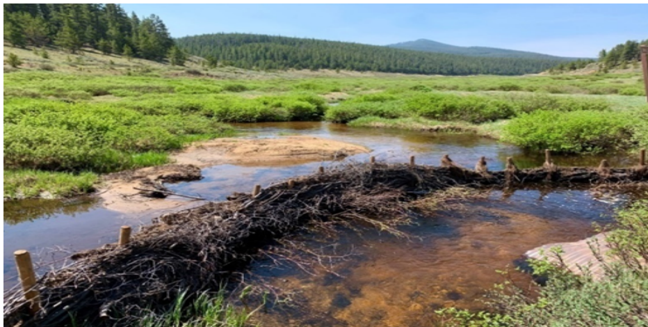
Photo by Jackie Corday of a starter dam built in 2022 with wood posts and interwoven willow branches on Trail Creek in the Gunnison National Forest in anticipation that beaver might block the culvert. It has been successful in protecting the culvert for over 3 years.
