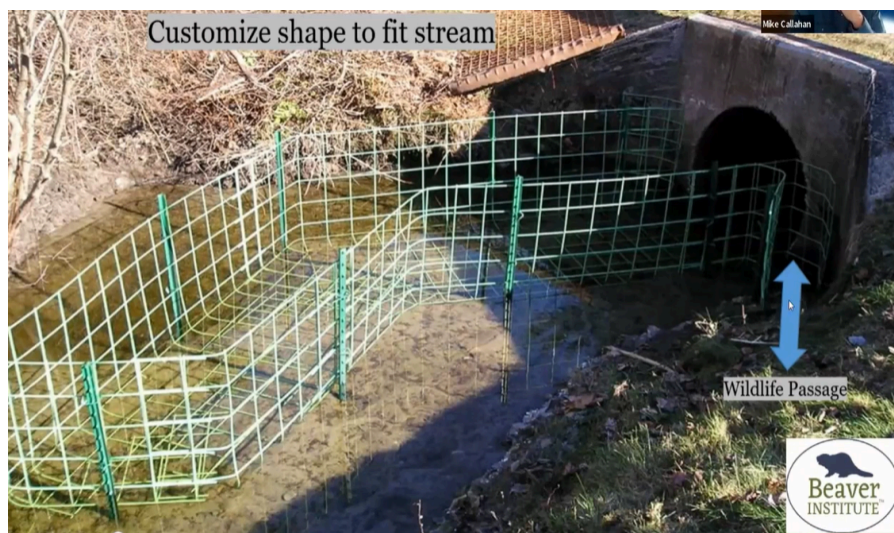
Photo from the Beaver Institute showing culvert exclusion fencing with a small stream and small culvert design with the blue arrow indicating an opening where wildlife can access the culvert to pass safely beneath the road.
