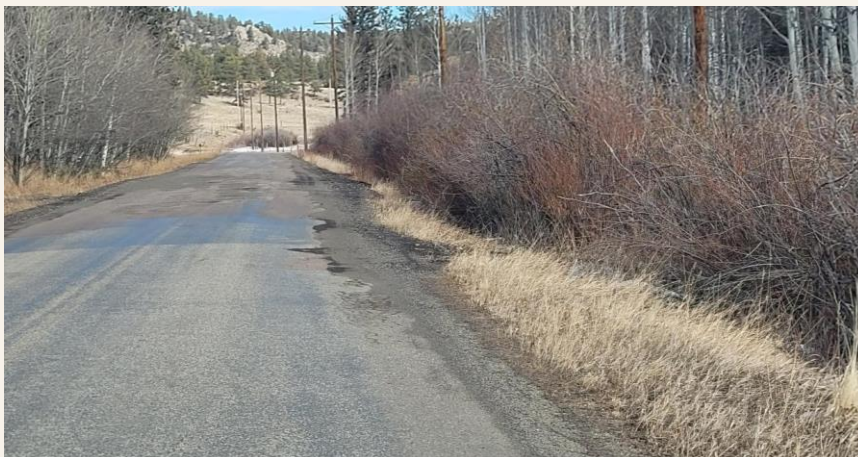
Figure 39. Road conditions at Eleven Mile State Park prior to the 2024 improvement project.
