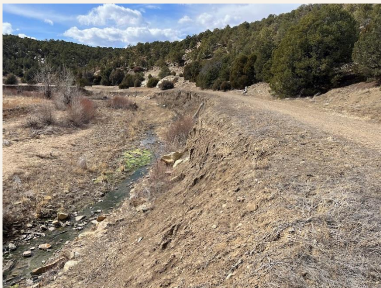
Figure 54. CR 18.3 near the Longs Canyon entrance. A major washout at this location has resulted in road closure since spring 2021 (photo taken spring 2024).
