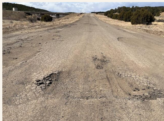
Figure 55. Unmaintained asphalt on CR 57.7 at the Reilly Canyon entrance.
