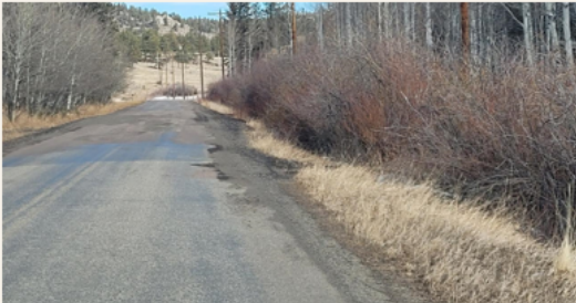
Figure 39. Road conditions at Eleven Mile State Park prior to the 2024 improvement project.
