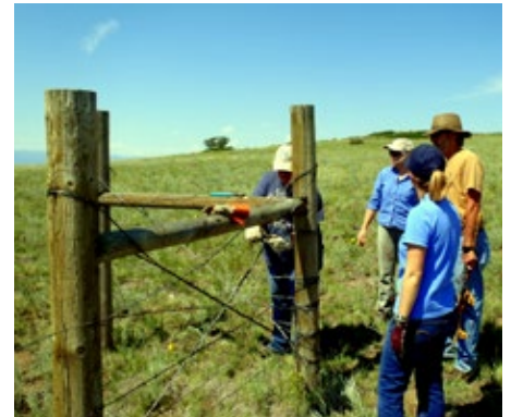
Staff, landowner, and volunteers repairing fence at High Mesa Natural Area, Fremont County
