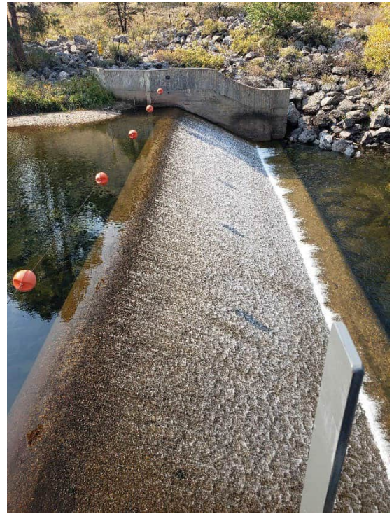
Figure 4-9. Fort Collins Intake at Gateway Park
