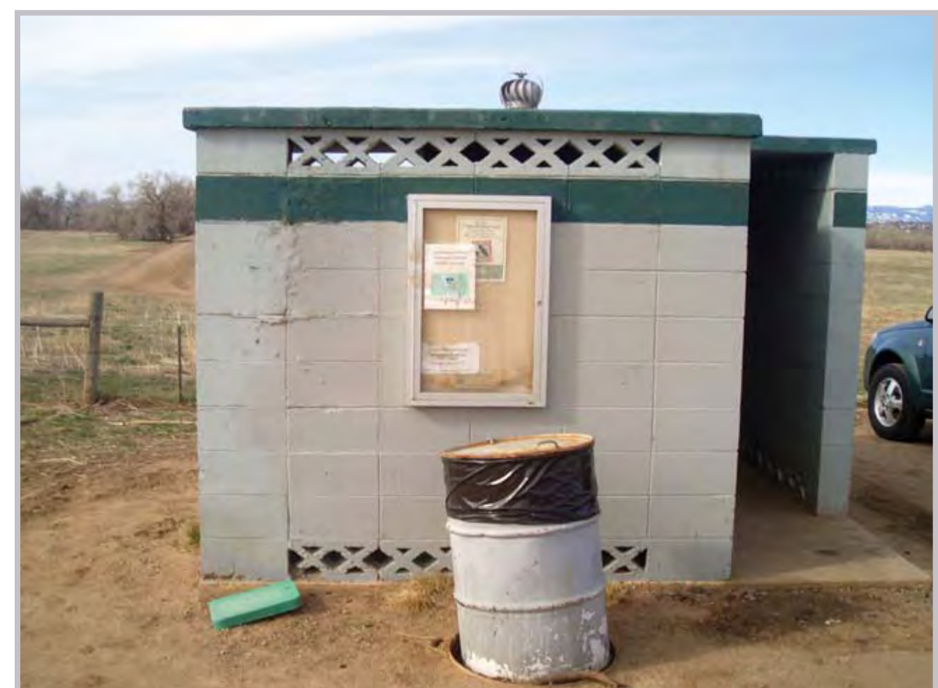
Dated restrooms and parking lots
