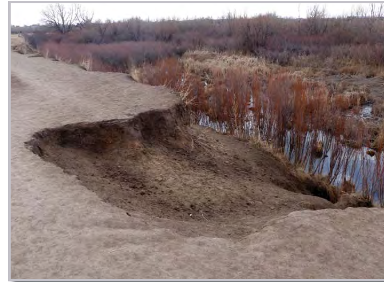
Trampled vegetation, erosion, and sedimentation
