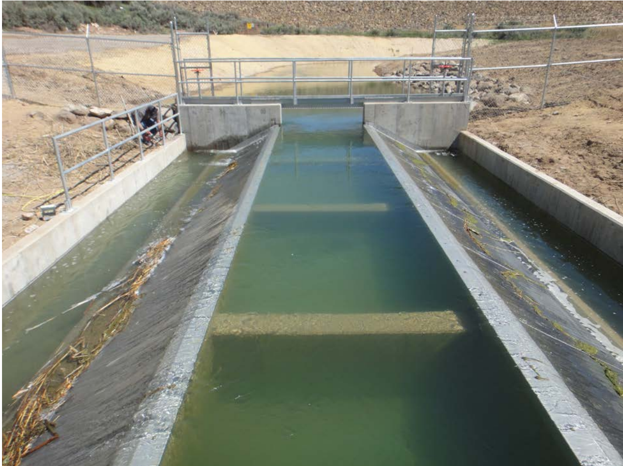
Figure 4. Rifle Creek fish screen looking upstream through structure.
