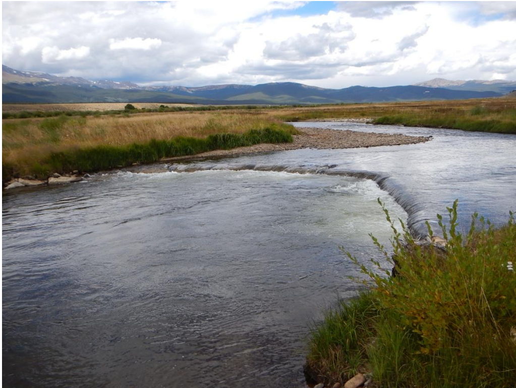
Figure 7.5. Typical log/rock-vane structure used during habitat restoration on the Upper Arkansas River.
