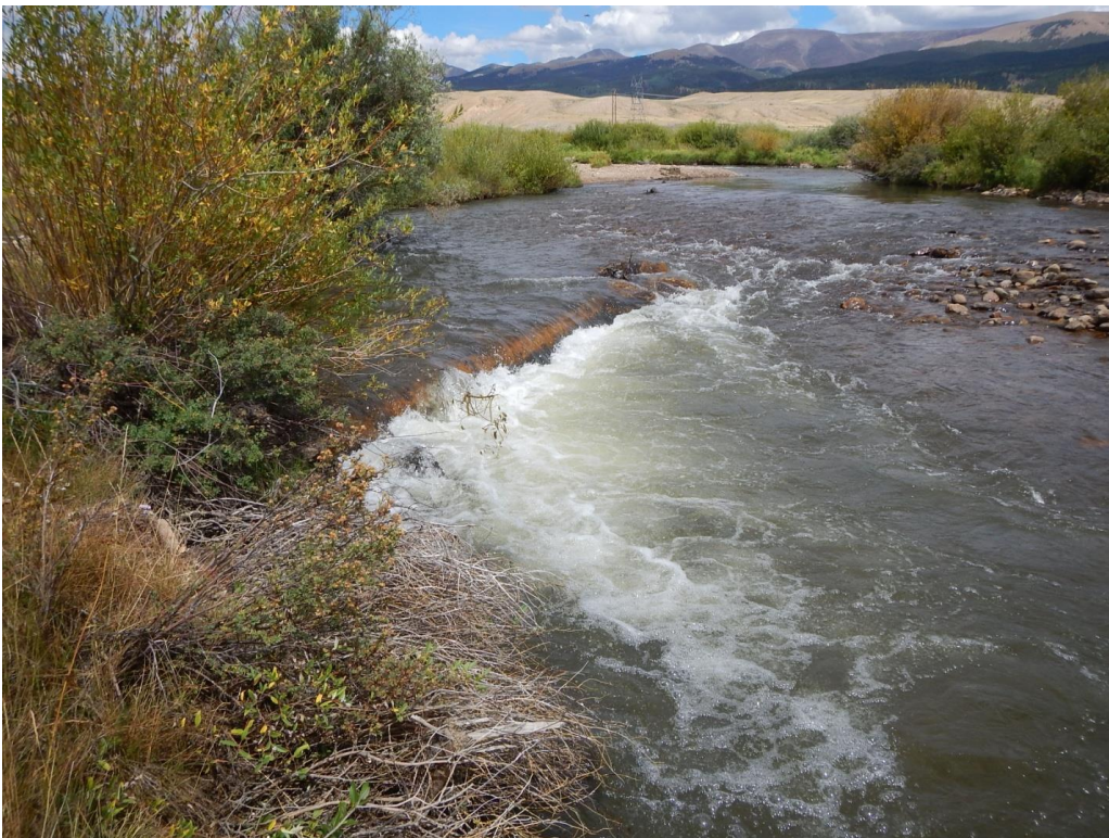
Figure 7.4. Typical log-vane structure used during habitat restoration on the Upper Arkansas River.
