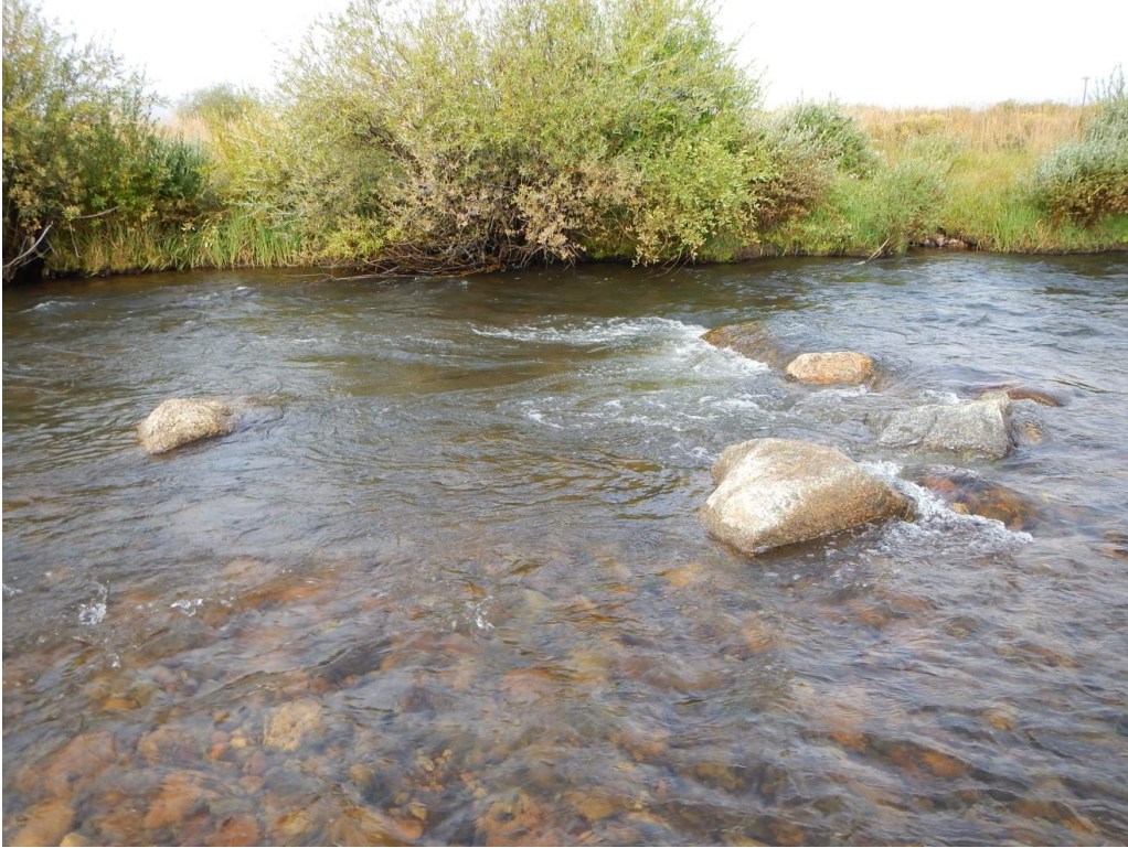
Figure 7.1. Typical boulder cluster structure used during habitat restoration on the Upper Arkansas River.
