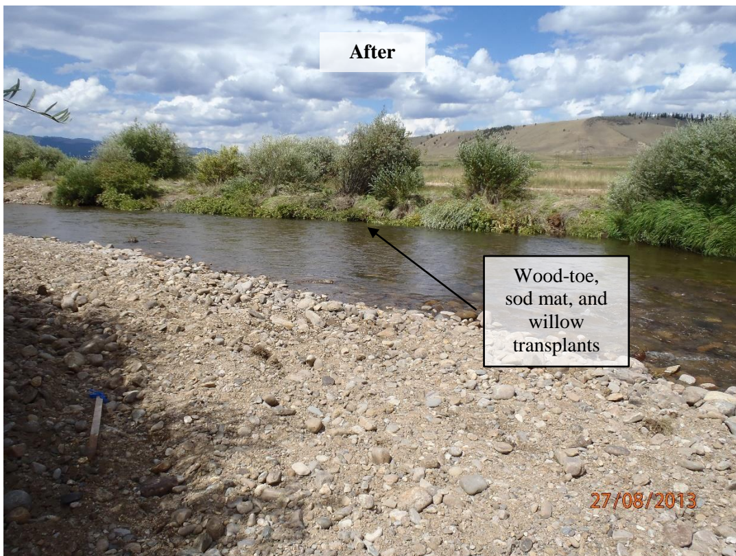
Figure 1.3. Before vs. after photos showing the treatment of excessive bank erosion with wood-toe, sod mats, and willow transplants on the Upper Arkansas River.
