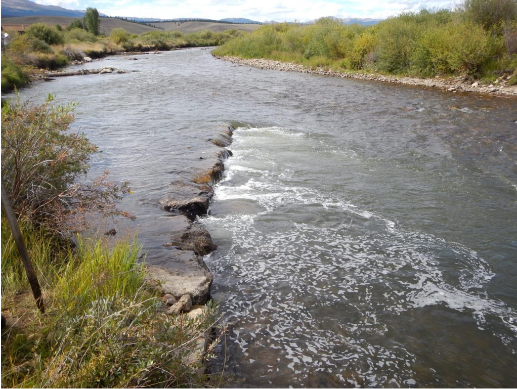
Figure 7.3. Typical rock-vane structure used during habitat restoration on the Upper Arkansas River.
