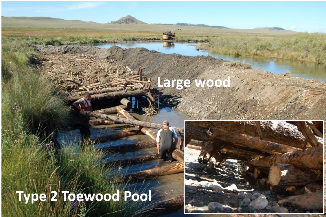
Figure 5. Type 2 toewood treatment during construction, consisting of an excavated pool, constructed point bar introduction of large wood at the bank toe to function as an undercut bank.
