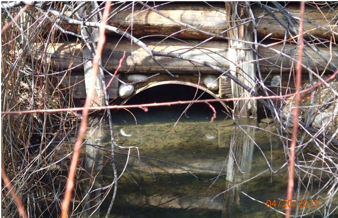
Figure 2. Outlet of the head gate culvert showing accumulation of sediment with adverse impacts on flows into the Piloni Ditch.
