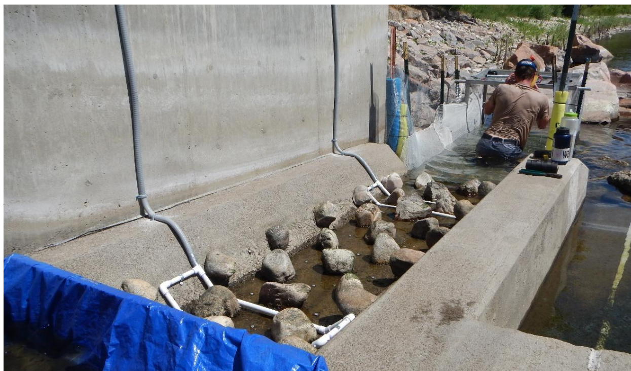
Figure 1. Picture of the rock-ramp fishway at the Fossil Creek Reservoir Inlet Diversion (FCRID) showing the location of PIT-tag antennae and the downstream enclosure.
