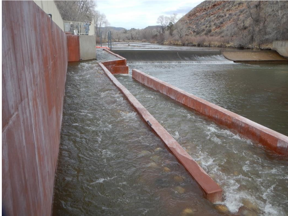
Figure 2.1. Engineering rock-ramp fish passage structure at the Watson Lake diversion structure on the Cache la Poudre River, Colorado.
