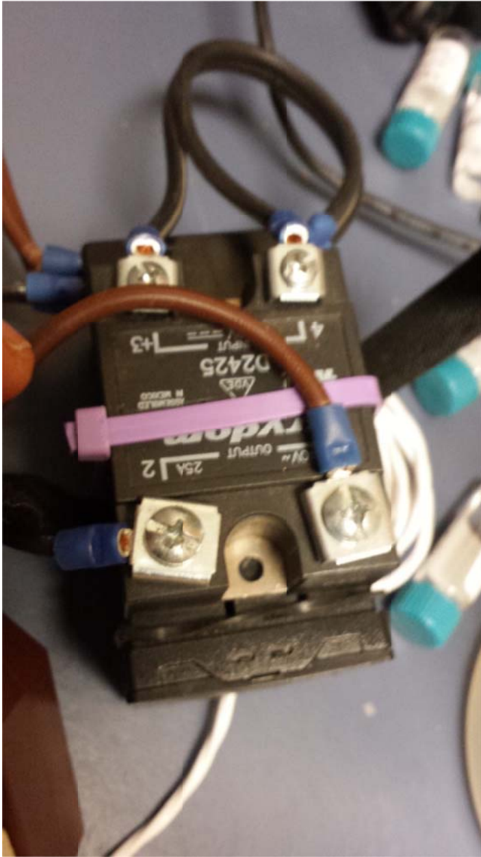
Figure 2.15- Crydom D2425 relay controlled by the Love brand temperature controller.
