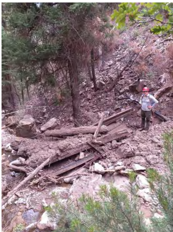
Remnants of Bridge #2 in stream channel
