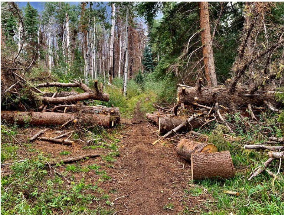
Upper left: tree clearing on Mansfield Ditch Trail, New Castle, WRNF, June 2022 Upper right and bottom left: tree clearing on Mill Creek Trail, Basalt Mountain, WRNF, June 2022
