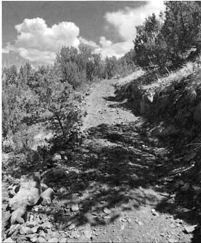
Section of trail at Penrose Commons that had been severely eroded, now rehabilitated with the RRMMC trail dozer and water diversion added to mitigate future damage.
