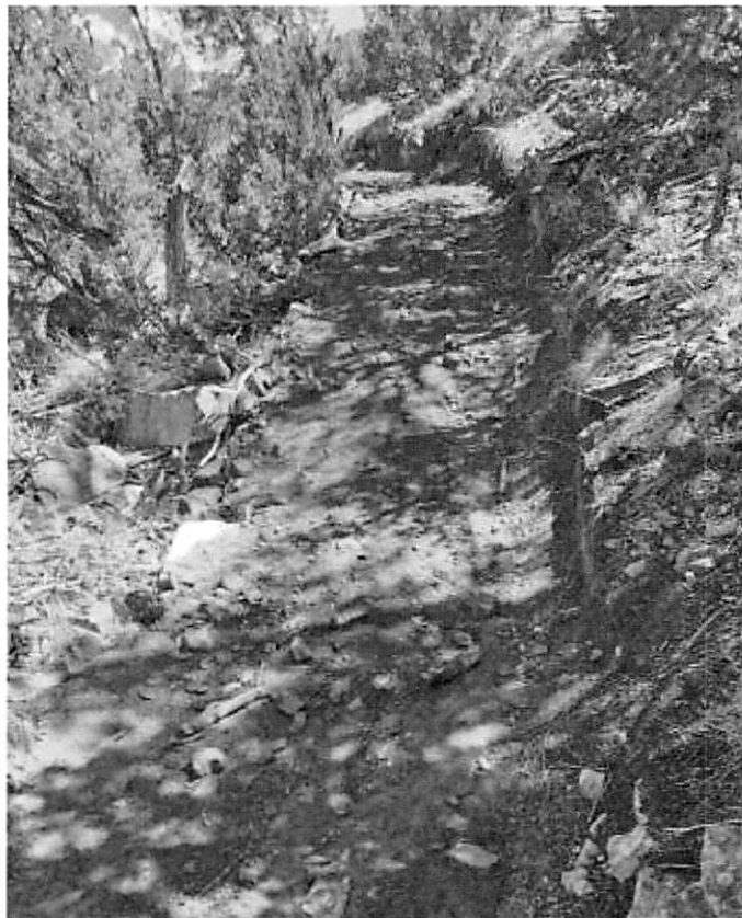
Section of trail at Penrose Commons that had been severely eroded, now rehabilitated with the RRMMC trail dozer.
