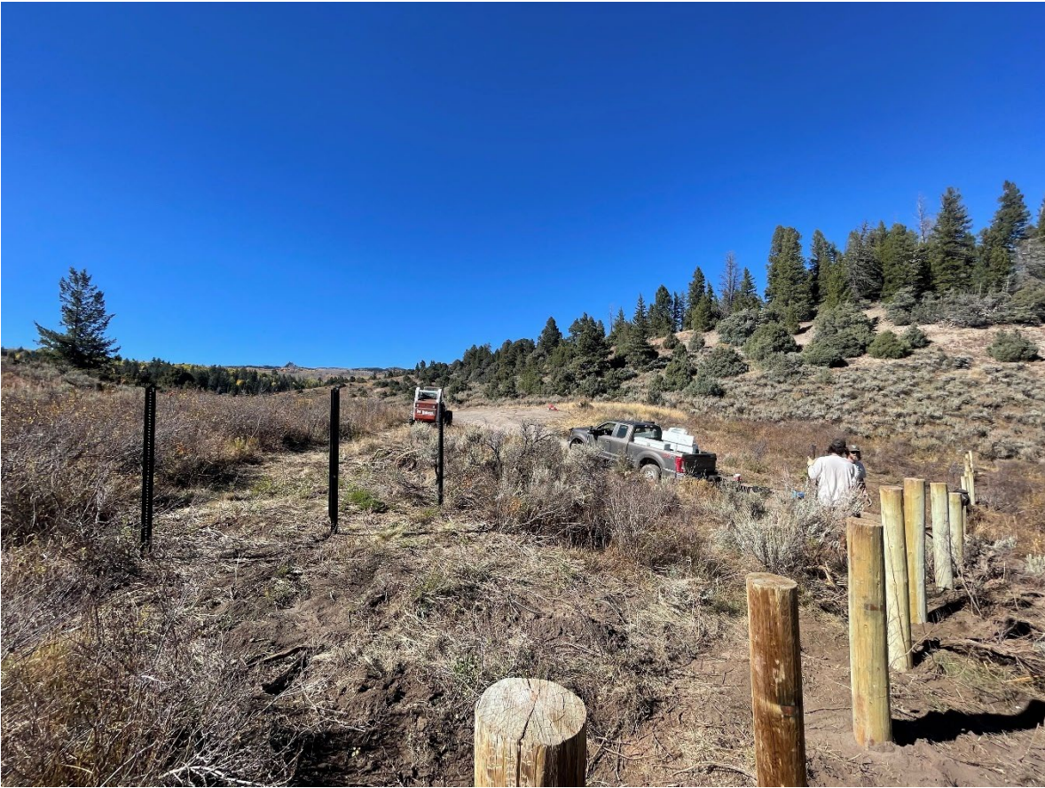
October 2023 – Here the OHV Crew is working to install barriers with the skid steer to protect the Blue Lakes area near the Castle Peak Wilderness Study Area (WSA). This area is a sensitive riparian area. The OHV routes surrounding Castle Peak are popular for BLM permitted OHV tours. Our permittees appreciate the work of the OHV Crew to keep routes labeled, maintained, and keep scenic areas like Blue Lake protected from damage.
